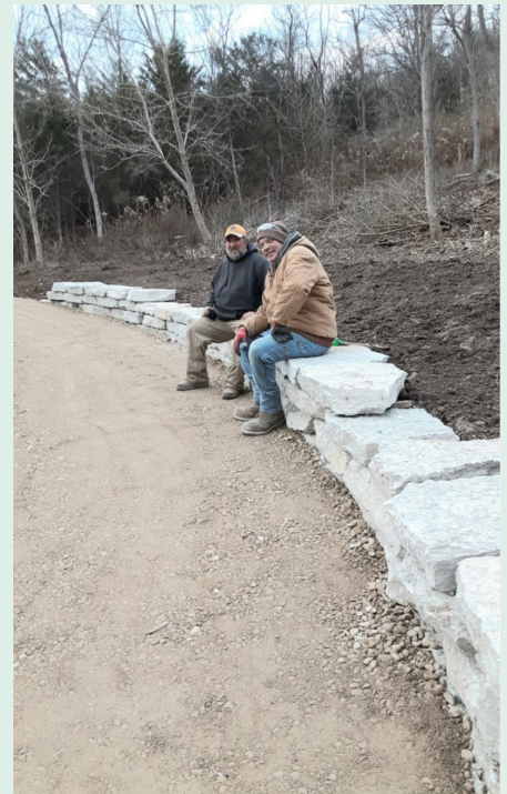
Prairie View Bench. A very special thanks to Jeffrey Allen Corporation and a great crew for going above and beyond in constructing our trail.
